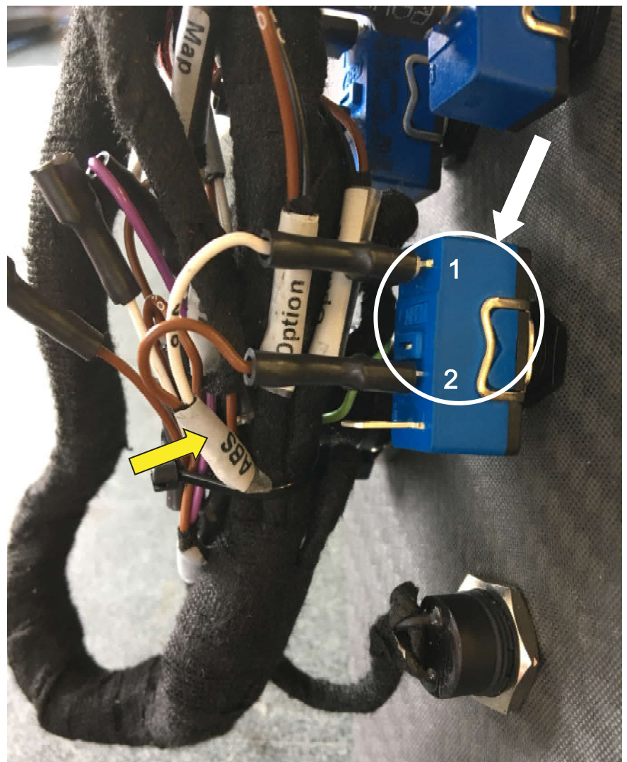
Step 22: Connection of the wet-dry switch to the wiring loom of the switch plate
