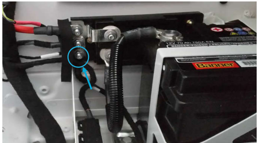
Detail: Connection point for the short cable piece to the battery disconnector
