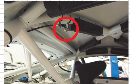
Figure 2.3 Three nozzles in the cockpit: #1 Roof
